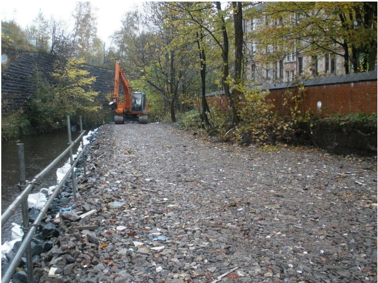
Photograph 2.1: Example of a raised working platform at White Cart Water FPS, Glasgow
